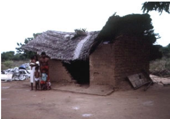
A house damaged by an elephant. The family narrowly escaped. One child was severely wounded by the falling bricks. Bundala
